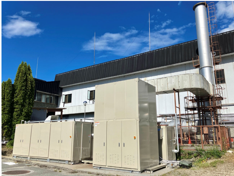
CO 2 separation and recovery equipment
