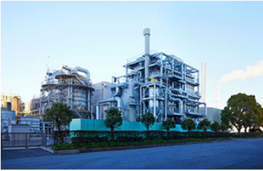
Biomass boiler (Chita Distillery)
