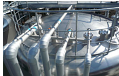
Reuse of water recycled at each stage of cleaning stored in 200-ton tanks
